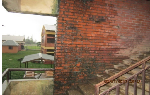
Figure1: Wall dampness during rainfall
