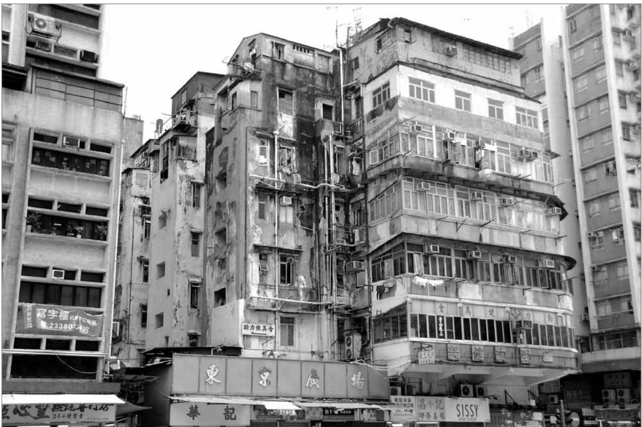
Figure 1: A dilapidated building in an old district in Hong Kong (photo: Daniel Chi Wing Ho).
